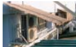
Awnings to shade outdoor air conditioner units realizes substantial energy savings.
