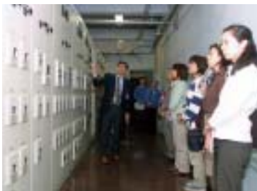
Explaining energy saving systems in front of centralized power management control panels
