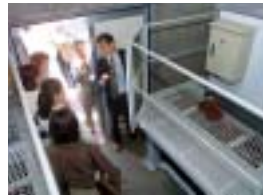
Air compressor room (see the illustration on the right)
